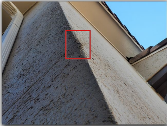
1- 2.5 Corner crack at the control joint
