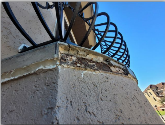
1- 5.1 Rusted drip edge flashing due to tiles
