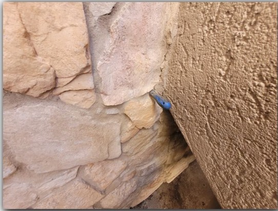
1- 1.5 Test Location P - Soft substrate encountered
