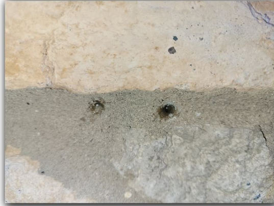
G- 2.2 Test holes in mortar
